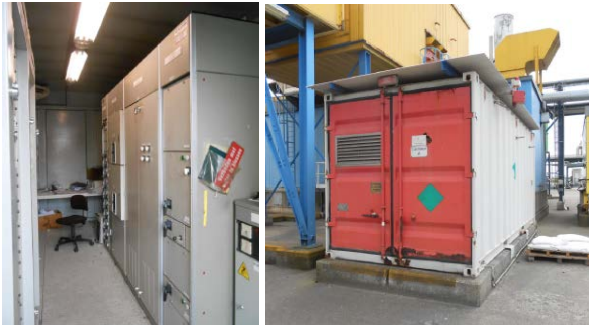
Inside view Electronic / electrical control cabinet
